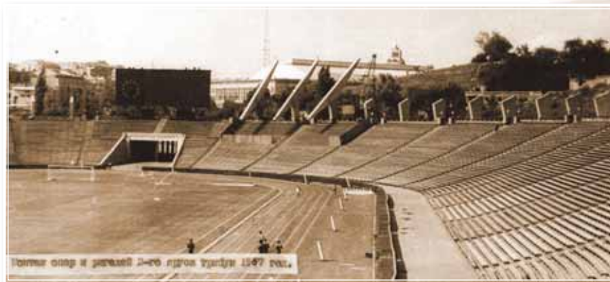
Installation of supports and bearers of the second tier of grandstands during the second general reconstruction of the Respublikansky Stadium. 1966
